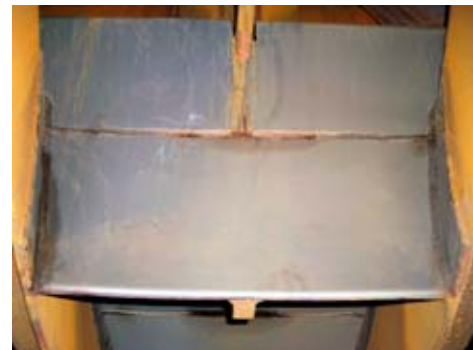
Figure 7. Wear on Fan B after Twelve Months in Operation
