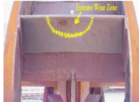
Figure 6. Wear on Fan A after Twelve Months in Operation
