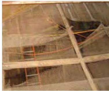
Stainless steel screens after less than 6 months performance.
